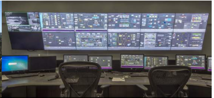
State of the art system controls, data acquisition (SCADA) and site security monitoring systems are centrally located in the LEED® Silver rated Administrative Building. Photo by Joel Grimes
