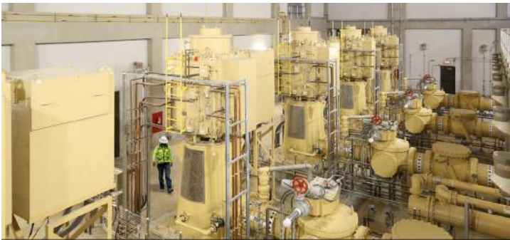
The raw water pump station houses five 375-foot (114 m) lifts, 12.5 MCD, 1,500 Hp vertical turbine pumps. Photo by Travis Bush
