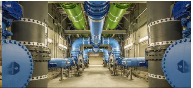
Pipe gallery in the filter building where raw water is filtered as part of the treatment process to produce clean water for the City of Austin. Photo by Joel Grimes
