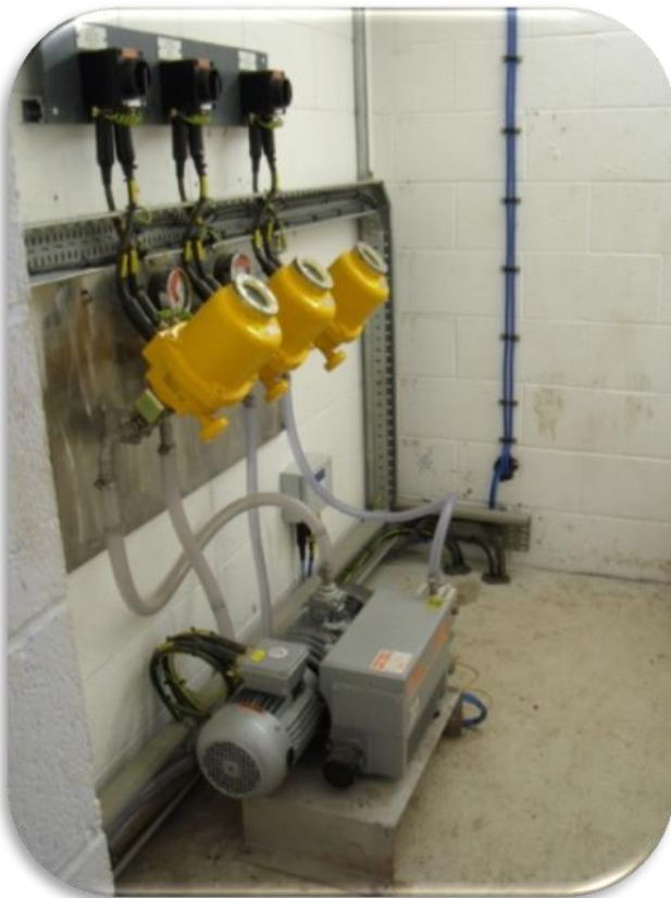
Figure 11: Vacuum Pump and Control Valves
