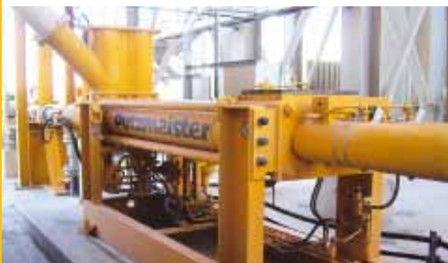
Plutonic gold mine, Australia: pumping of gold mine tailings
