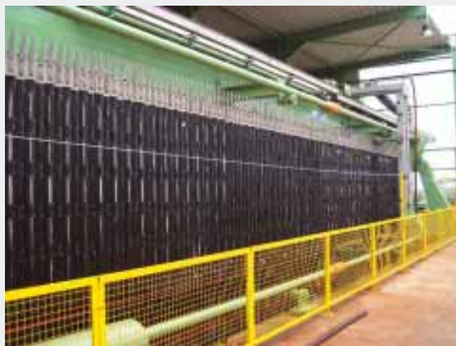
A series of filter presses dewater the tailing materials
