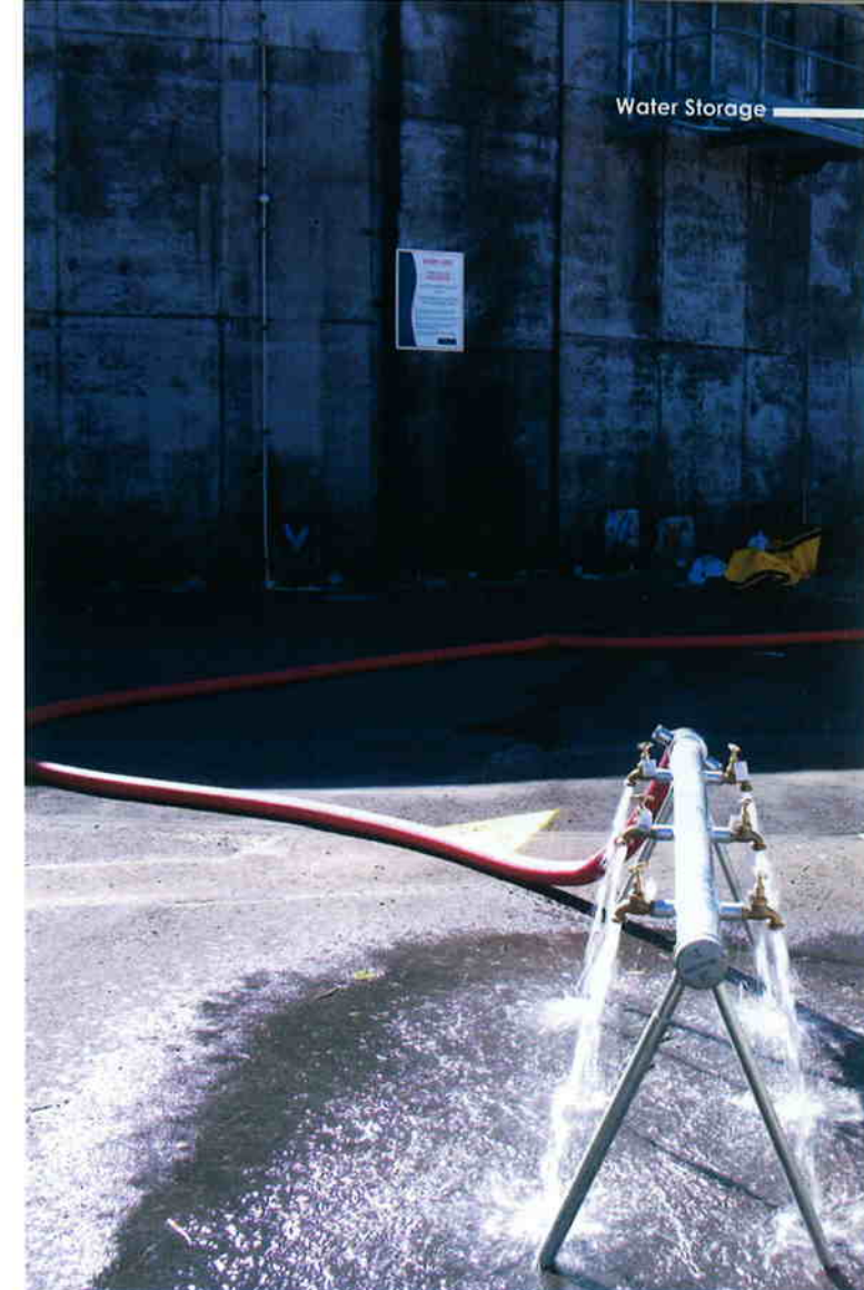
Figure 2 -- Capacity Emergency Manifold Stand at Reservoir
