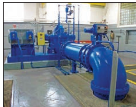
Figure 9. High-Service Pump No. 7.
