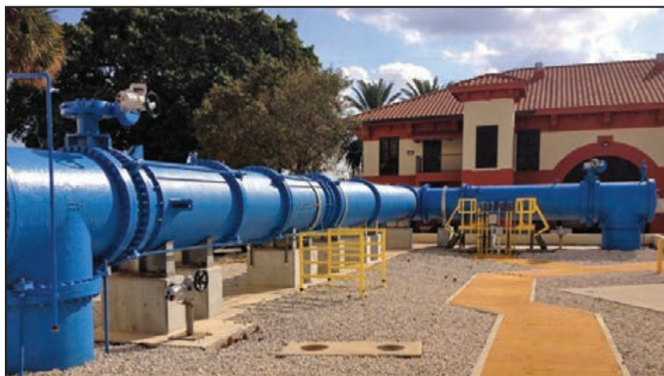
Figure 6. Mixing and Metering Header.
