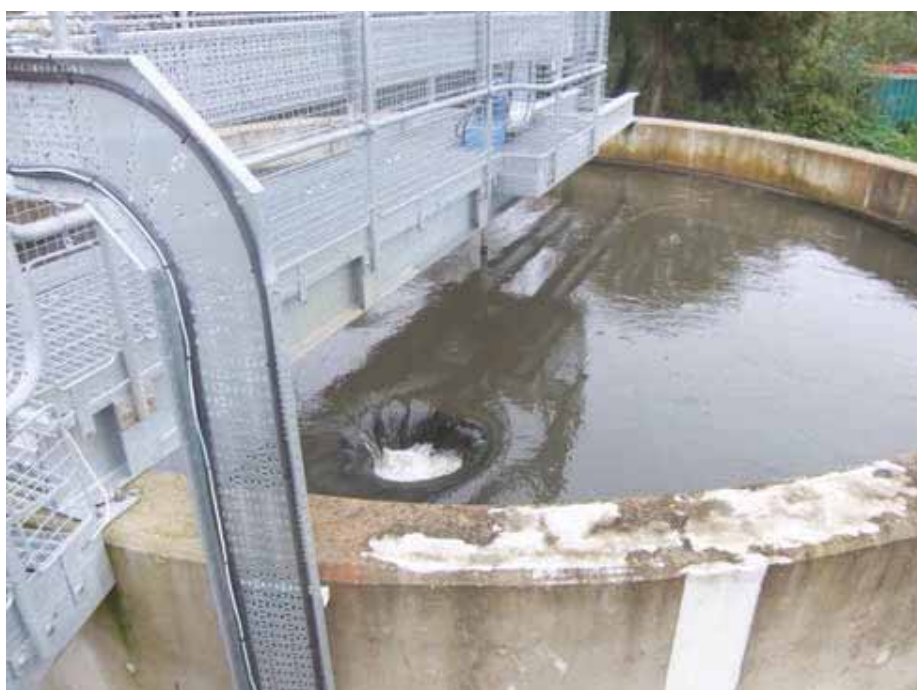
Chemical dosing and flocculation improve filter performance. Photo by MWH
