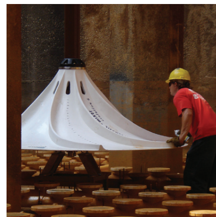
Hypermixers being installed in Washington DC, USA
