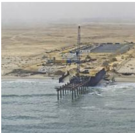
AREVA, inaugurated the very first sea water desalination plant in Namibia, located 30 km north of Swakopmund on the Atlantic coast. The plant will produce 20 million m 3 of potable water per annum, which is enough to allow AREVA to operate the Trekkopje mine without pumping any water from boreholes. Excess production serve local communities and industrial activities
