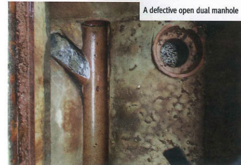
Ragging from an outfall discharging into Alexandra Park Stream
